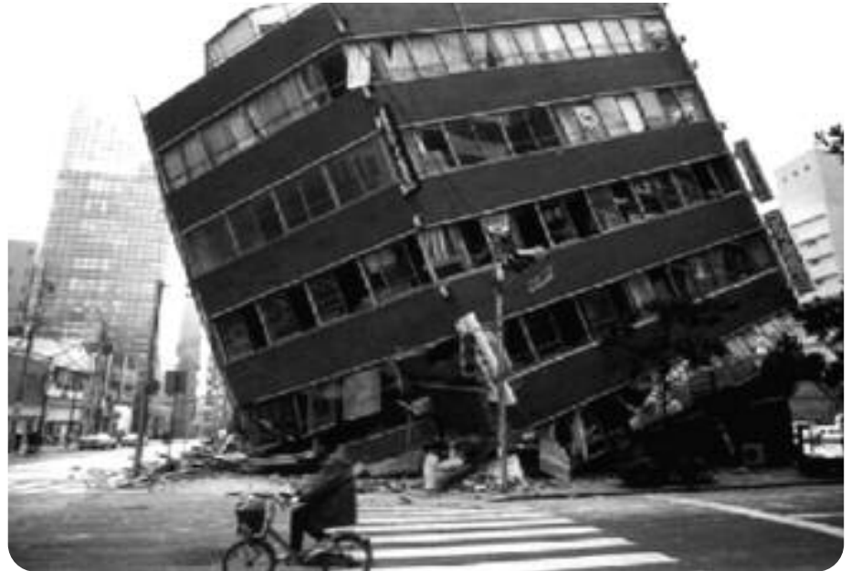
Kobe after the quake. Source: www.niksula.cs.hu.fi/~haa/kobe.html
